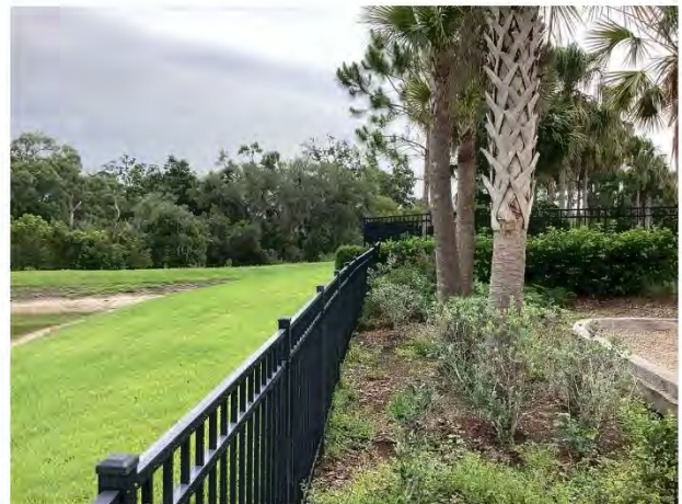
Fence leaning section
