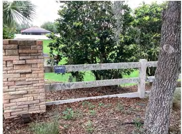
Fence finish deterioration
