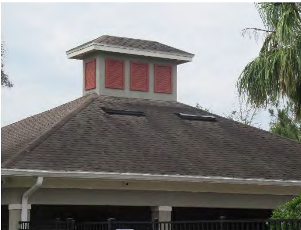
Clubhouse asphalt shingle roof (note weathering)
