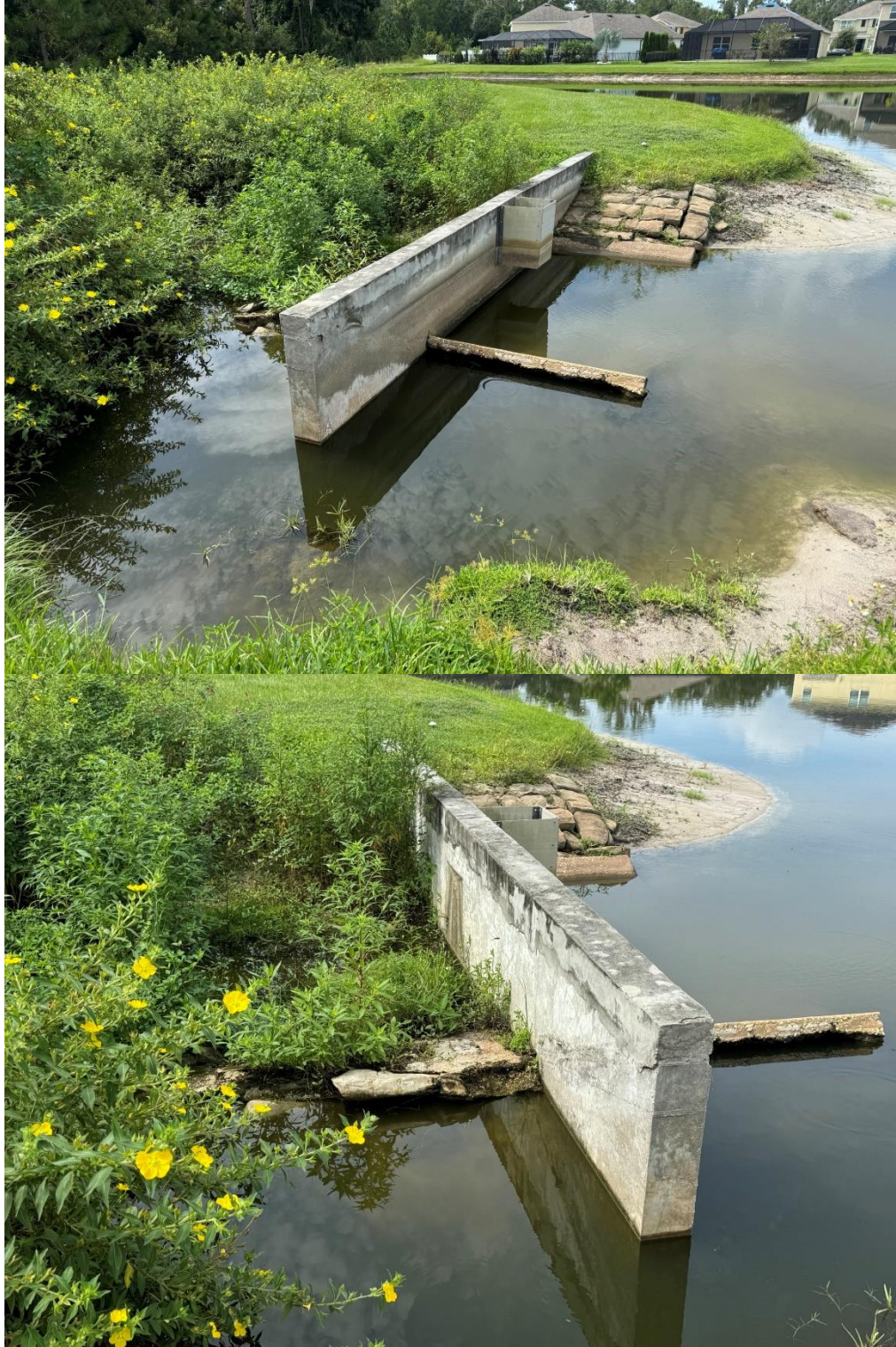
Photo 3 – Displays the washed-out control structure at Pond H. The structure was observed to be intact, but due to the overgrowth that will need to be determined during the repair.
