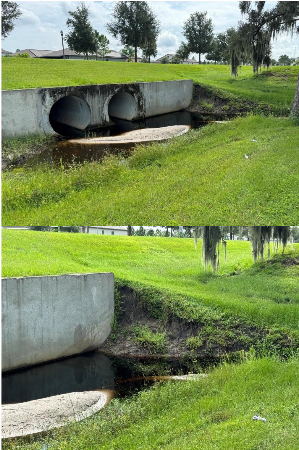
Photo 4 – Displays erosion and sediment deposits on the downstream end of the dual 60" storm water pipes that run under Silverado Ranch Blvd. The erosion appears to be from when the control structure at Pond H failed.
