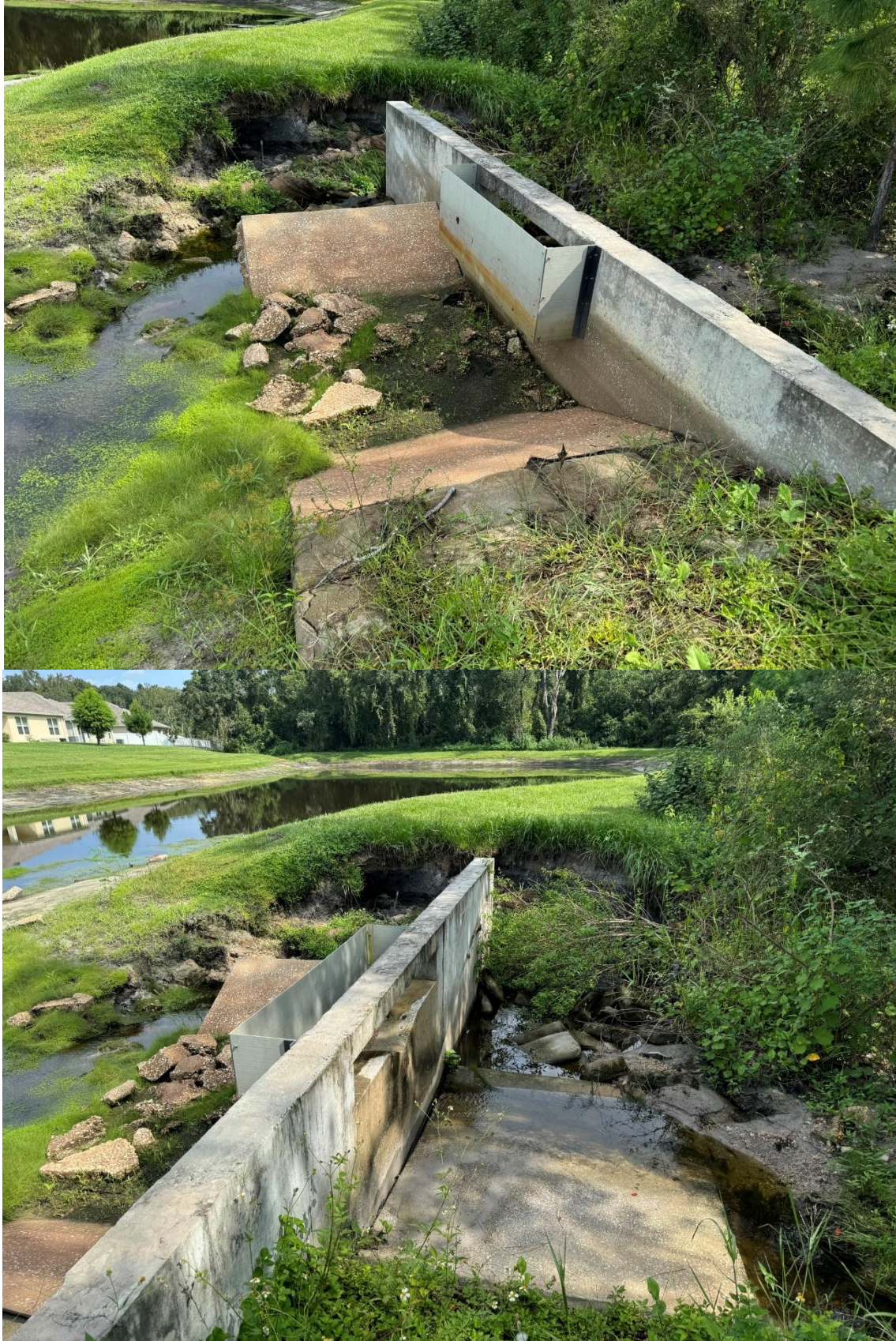
Photo 1- Displays the washed-out control structure at Pond J. The ditch paving on the back side of the weir has slumped due to increased erosion.
