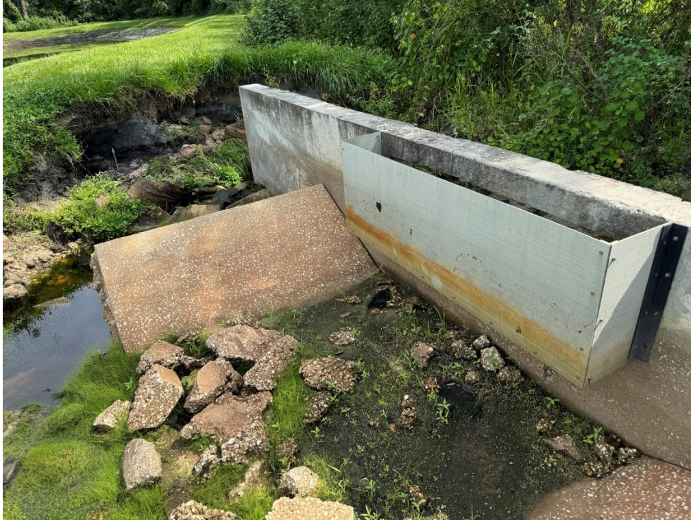
Photo 2 – Closer view of the erosion on the NE bank.
